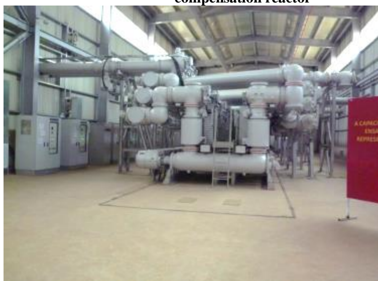
Figure 7-17 Indoor type gas-insulated switchgear
