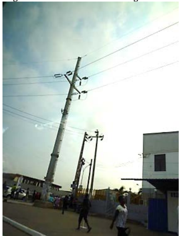
Figure 7-8 60 kV steel pipe tower
