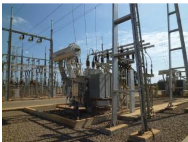
Figure 7-14 66 kV/15 kV transformer made in China
