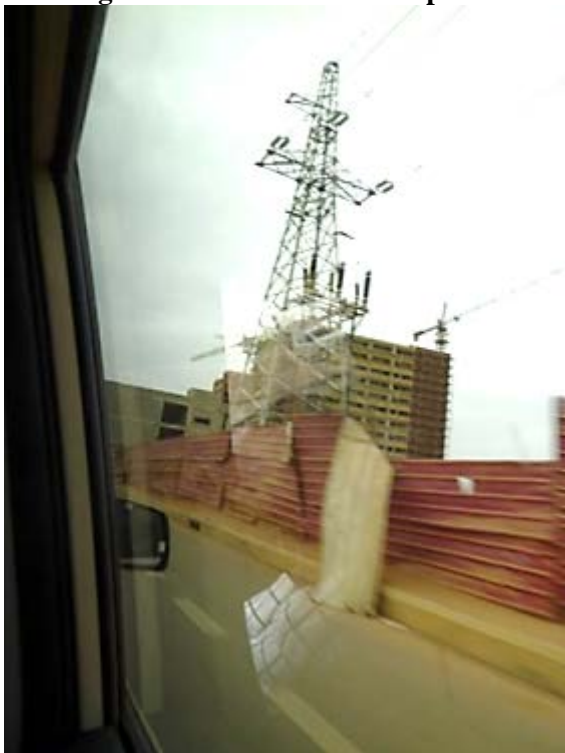
Figure 7-7 60 kV underground cable branch tower
