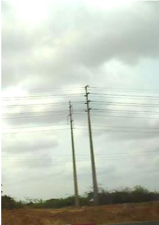
Figure 7-5 66 kV concrete pole
